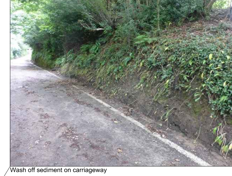
Wash of sediment on carriageway
