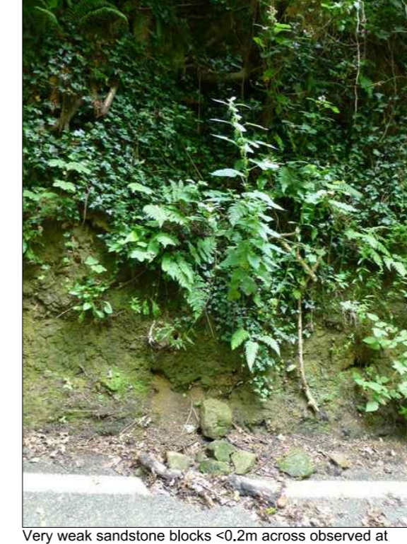
Very weak sandstone blocks 0.2m across observed at the edge of the carriageway from surface failure above
