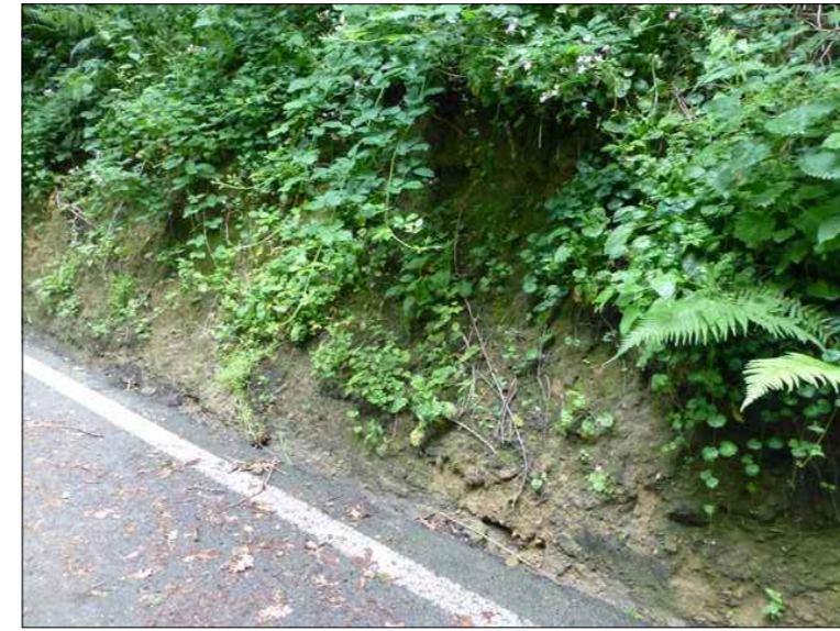
Low level shallow surface slip
