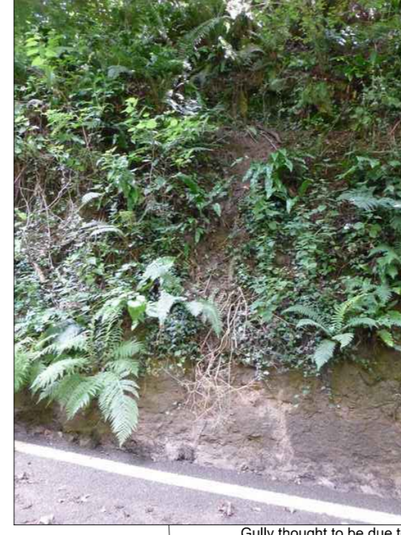
Gully thought to be due to concentrated surface water flow
