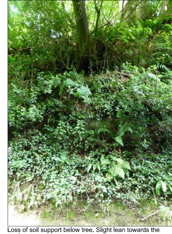
Loss of soil support below tree. Slight lean towards the carriageway
