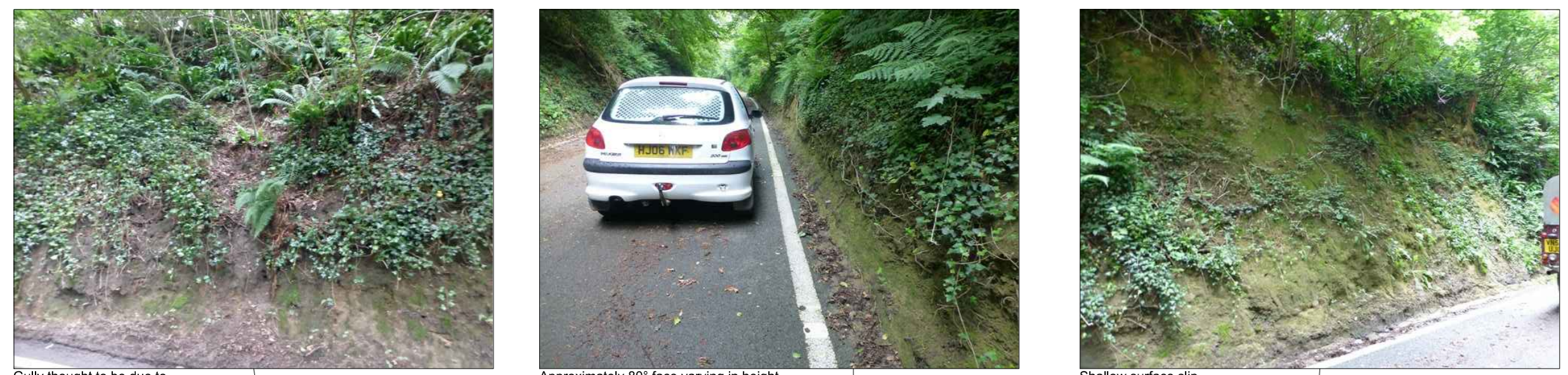
Gully thought to be due to concentrated surface water flow
