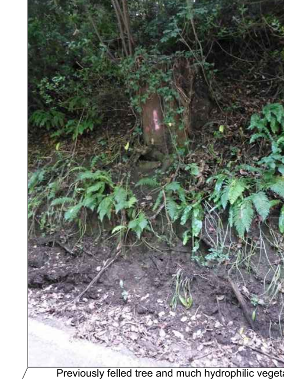
Previously felled tree and much hydrophytic vegetation. Future decomposition of the stump may lead to loss of soil support and subsequent slope failure
