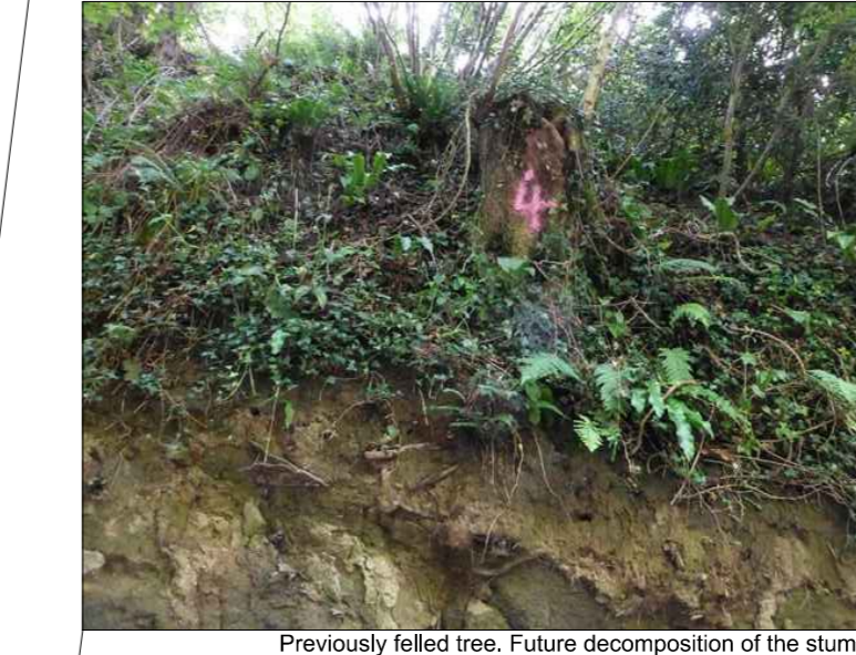
Previously felled tree. Future decomposition of the stump may lead to loss of soil support and subsequent slope failure
