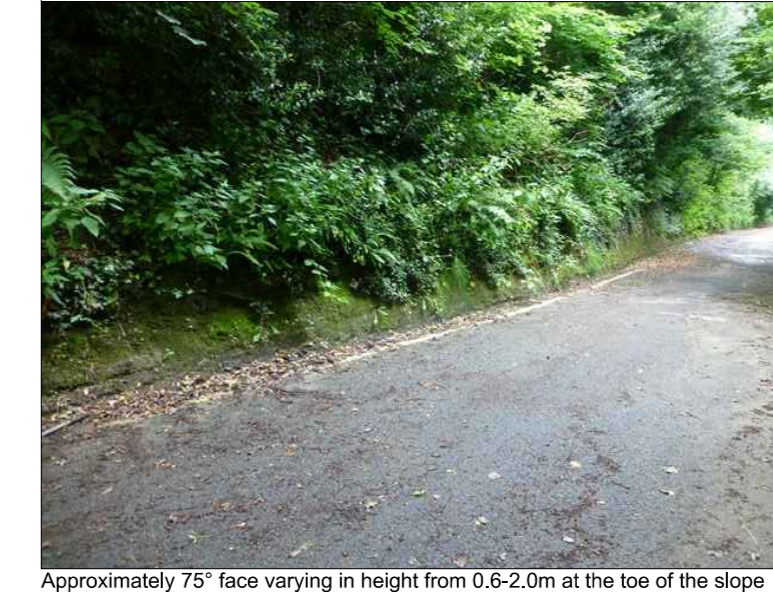
Approximately 75° face varying in height from 0.6-2.0m at the toe of the slope
