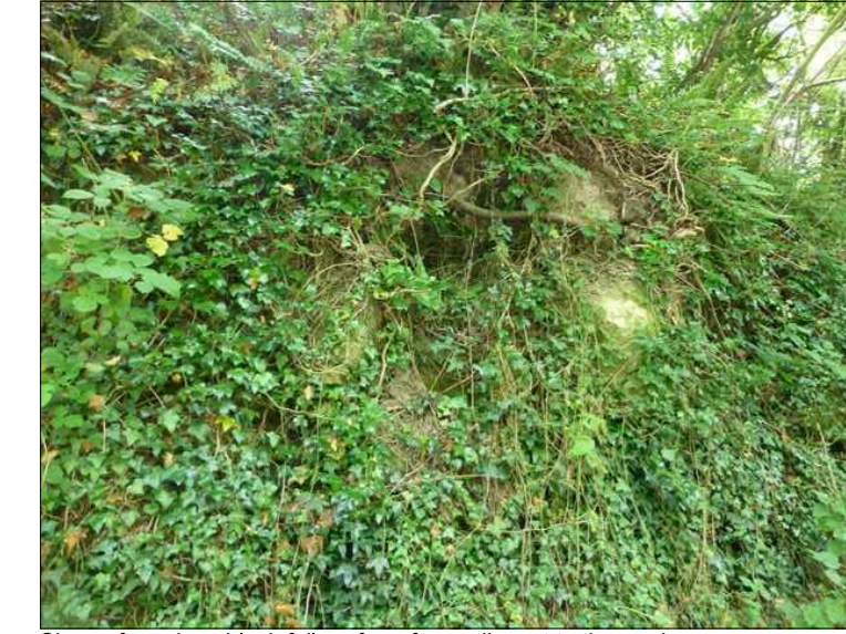
Signs of previous block failure from face adjacent to the carriageway
