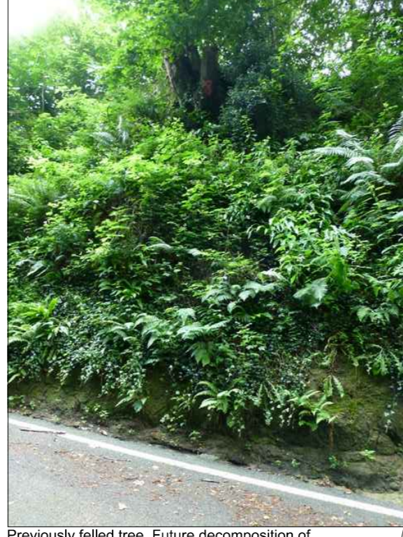
Previously felled tree. Future decomposition of the stump may lead to loss of soil support and subsequent slope failure
