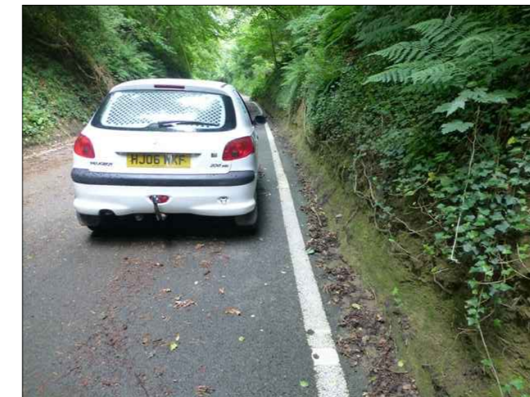
Approximately 60° face varying in height from 0.25-1.6m at the toe of the slope
