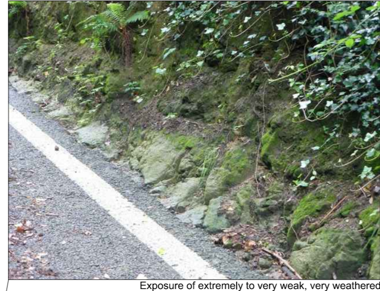
Exposure of extremely to very weak, very weathered sandstone from road level to 1.3m above the carriageway
