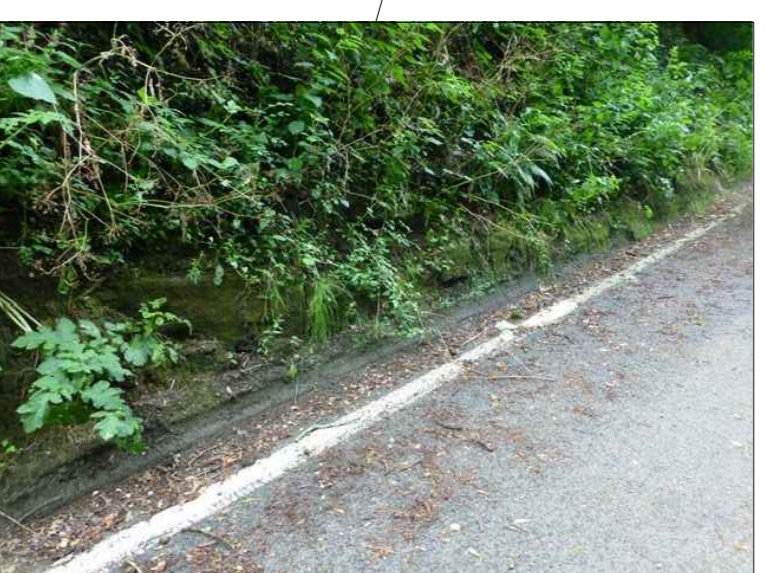
Exposure of extremely to very weak, weathered sandstone from road level to 1.5m above the carriageway
