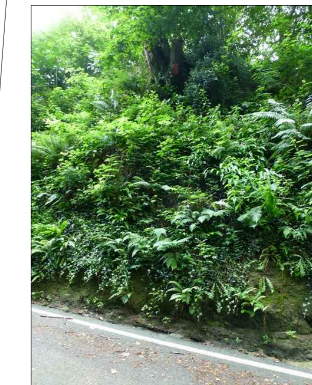
Previously filled tree. Future decomposition of the stump may lead to loss of soil support and subsequent slope failure
