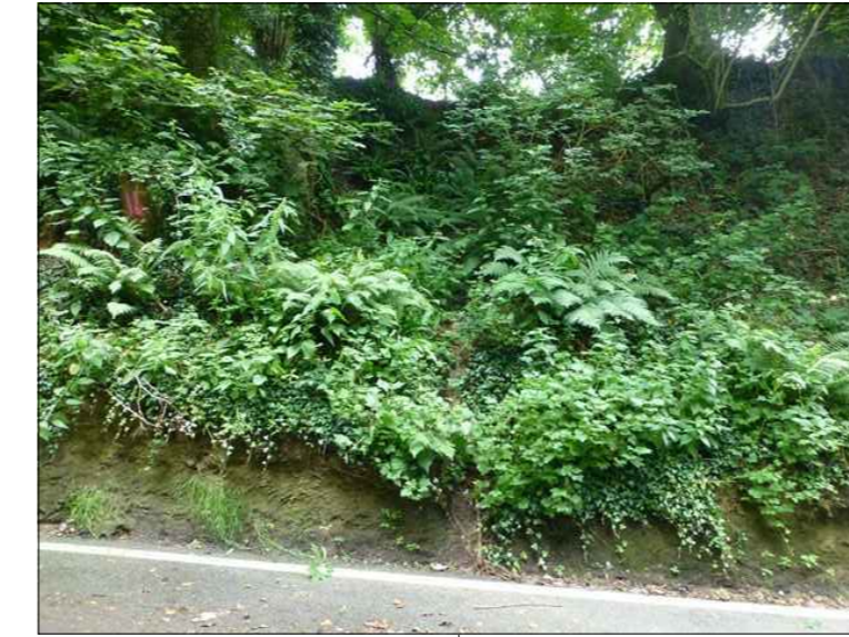
Gully thought to be due to concentrated surface water flow
