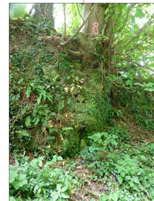
Overhanging rock blocks on face adjacent to the carriageway
