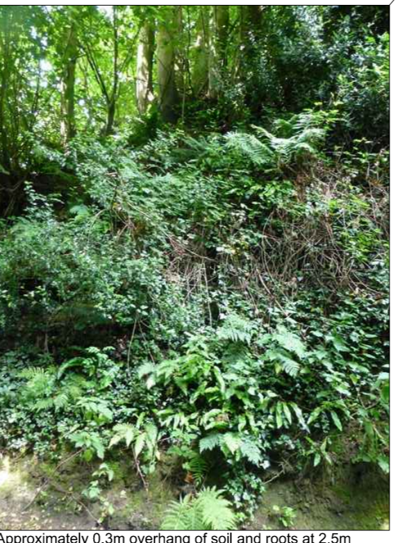
Approximately 0.3m overhang of soil and roots at 2.5m above the carriageway
