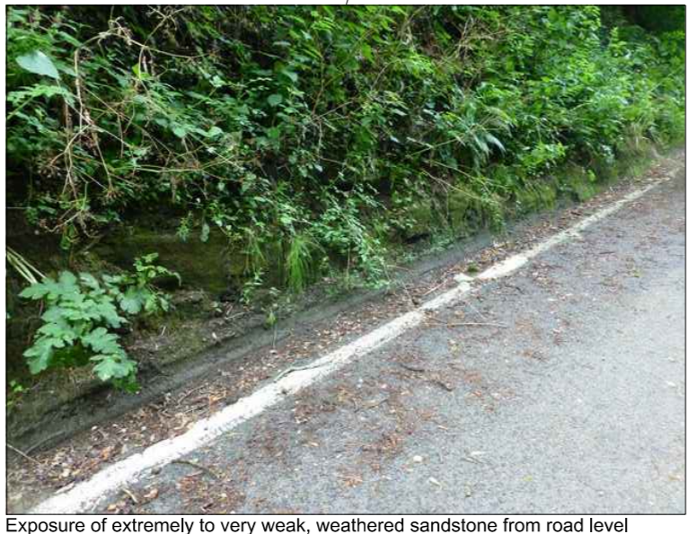
Exposure of extremely to very weak, weathered sandstone from road level to 0.5m above the carriageway
