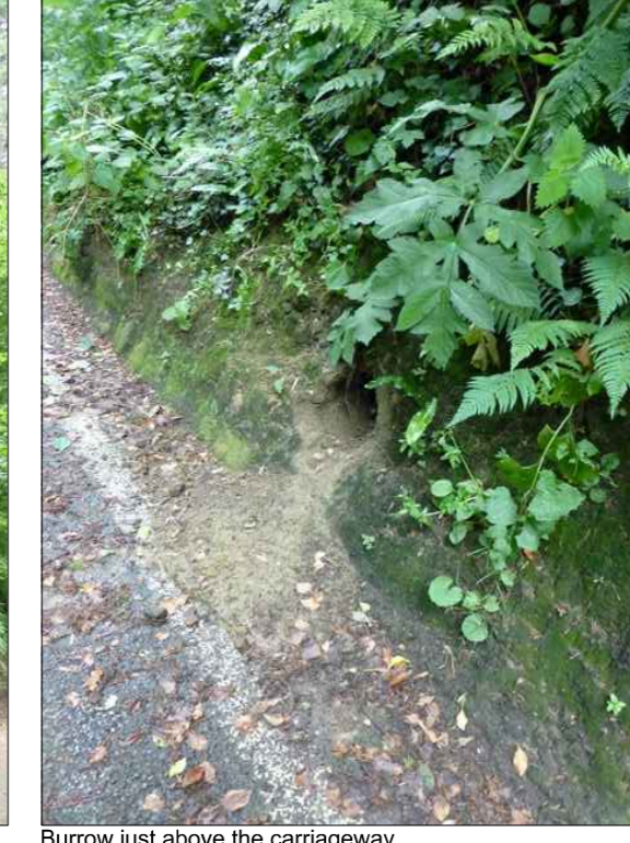
Burrow just above the carriageway
