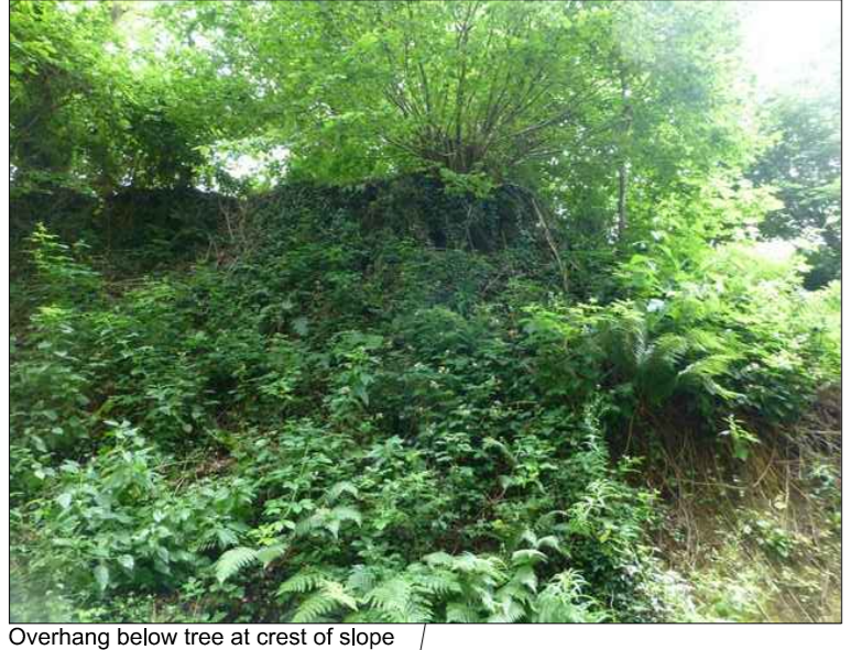
Overhang below tree at crest of slope
