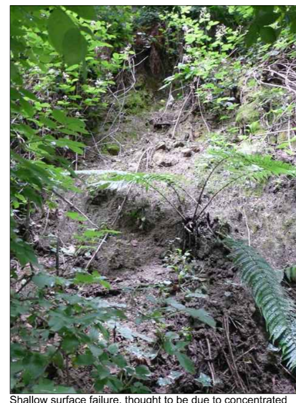
Shallow surface failure, thought to be due to concentrated surface water flow. Failed material observed on the carriageway
